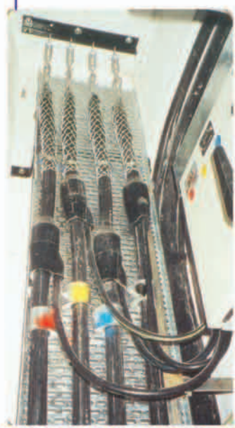
Cable brackets and terminals
