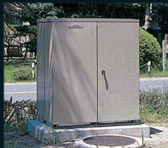
構内の設置例 INSTALLATION CASE IN CAMPUS
