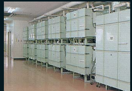
信頼性を高く維持する厳密な品質チェック装置 STRICT QUALITY CONTROL EQUIPMENT MAINTAINING THE HIGH RELIABILITY OF OUR PRODUCTS
